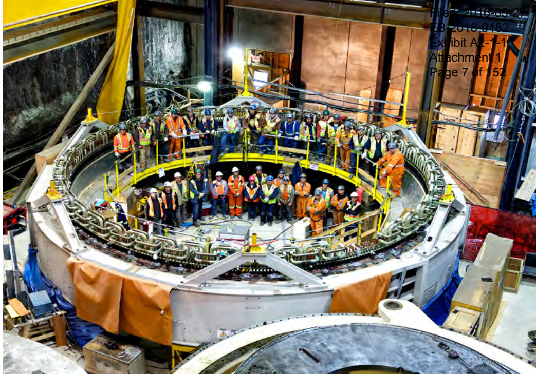
Interior of the new Smoky Falls generating station, Lower Mattagami Project.
