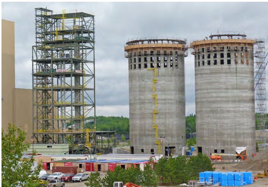
Biomass silos at the OPG's Atikokan thermal generating station.
