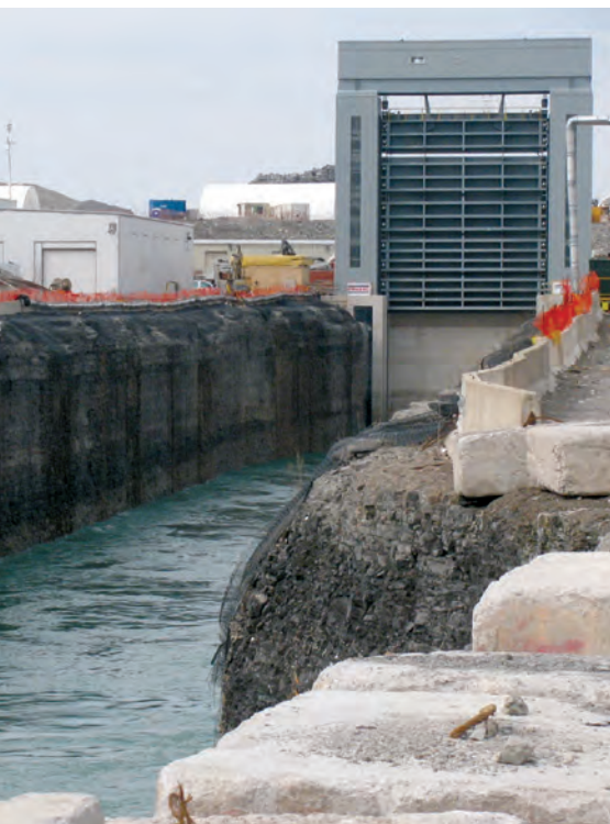
The new Niagara Tunnel outlet tunnel and gate will provide more, clean, renewable power for Ontario.
